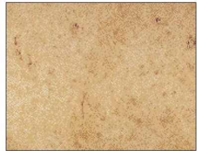
304 PERFORMANCE AFTER 20 YEARS SERVICE IN MEDIUM TO SEVERE MARINE ENVIRONMENT
