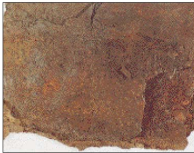
MILD STEEL PERFORMANCE AFTER 5 YEARS SERVICE IN MEDIUM TO SEVERE MARINE ENVIRONMENT
